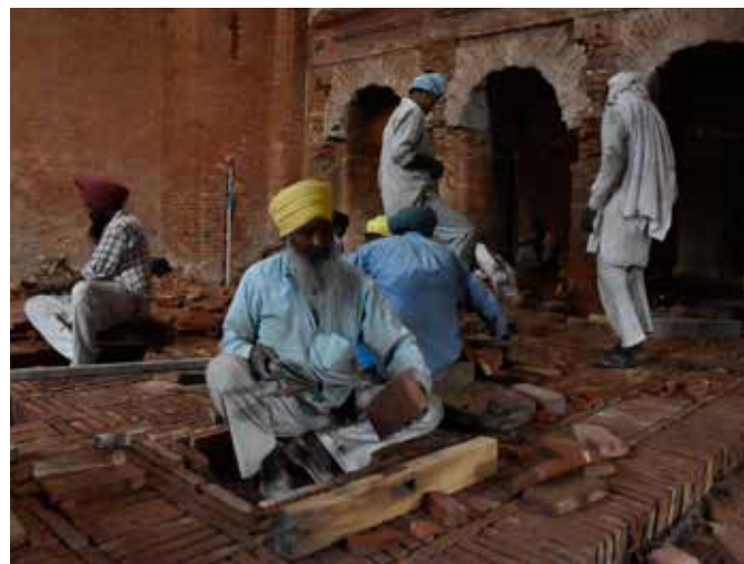
Flooring in brick tiles as part of conservation of the interiors of the Rambagh Gate
