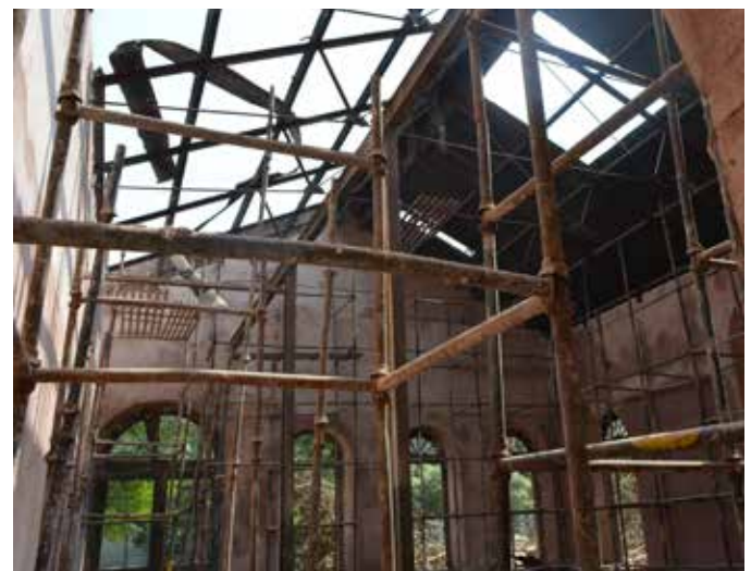
Internal view of the dismantled roof of the pump house at 40 Khoo while conservation is underway
